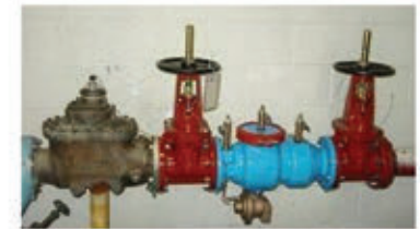
Newly Installed 4-Inch Reduced Pressure Principle Backflow Preventer
